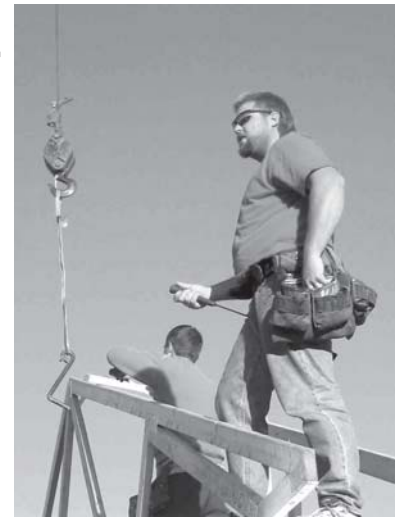
Duane and Julia Sauter owners of Sauter Construction brought some friends out and put up the Clawson trusses at the Busbys' home.
